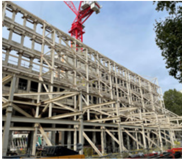
A reuse steel project in Holbein Gardens, London – Cleveland Steel & Tubes Ltd
