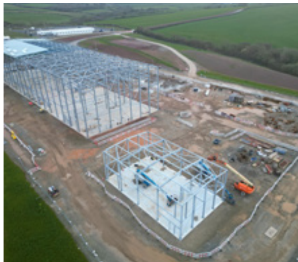
Pembroke Converter Station, South Wales - Shipley Structures Ltd
