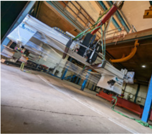
Installation of Ficep Kronos system at John W. Laycock – Ficep (UK) Ltd
